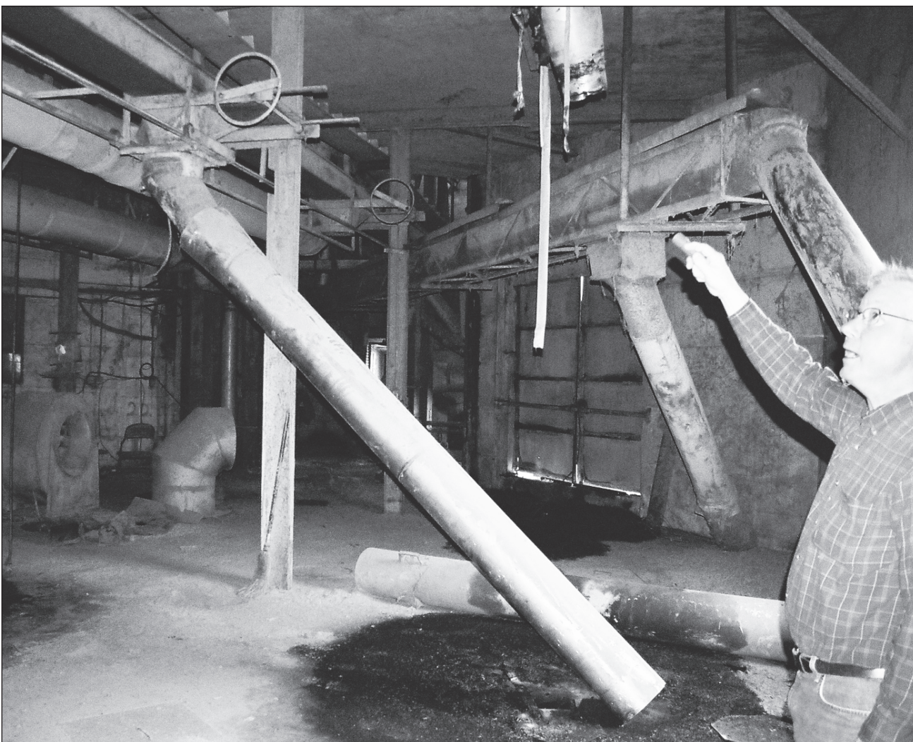
These pipes could be moved around to flow the rice into the various bins below for storage. Metal plates on the floor were opened to access the bins.
