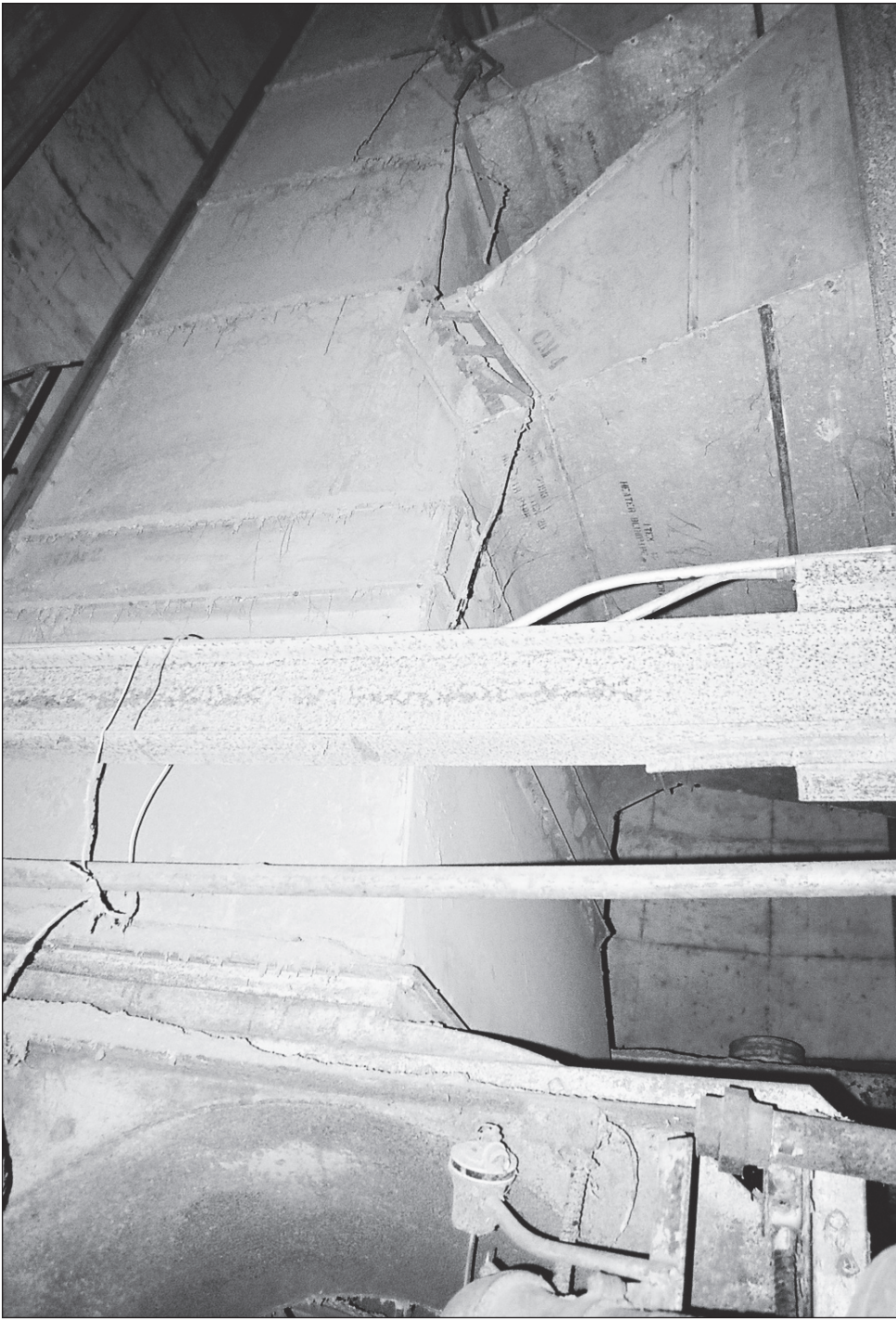
This is the main dryer structure, viewed from the bottom. Note the three graduated ducts going off to the right.
